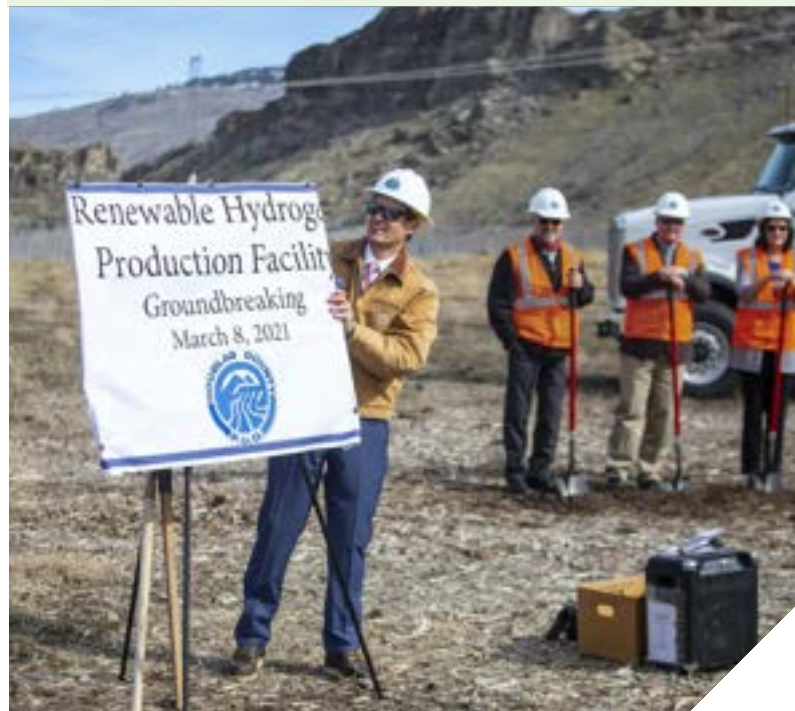
Douglas County Public Utility District General Manager Gary Ivory, holding a sign in the foreground, says the renewable hydrogen facility should be operating at the end of the year at this site in a former apple orchard near East Wenatchee. PUD commissioners are in the back ready with shovels. From left, Ron Skagen, Aaron Viebrock and Molly Simpson.
